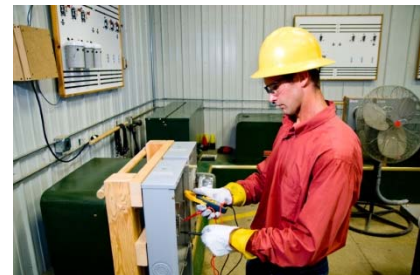
Worker testing the wiring on equipment to ensure the equipment is deenergized
