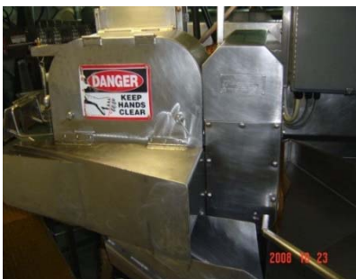
Guard with appropriate signage
