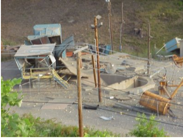
Figure 2. Damaged Surface Facilities
