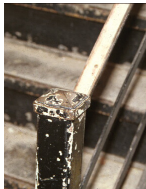
FIGURE 12.5 A metal railing before abatement.
