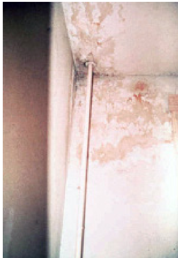
FIGURE 13.2 Deteriorated paint on surfaces that are unsuitable for encapsulation
