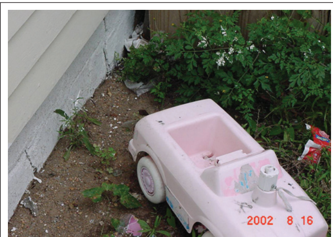
FIGURE 5.9 Soil lead hazard at dripline
