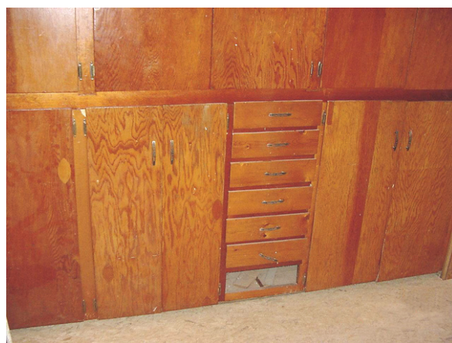
FIGURE 15.10 Surfaces that may have had paint stripped.
