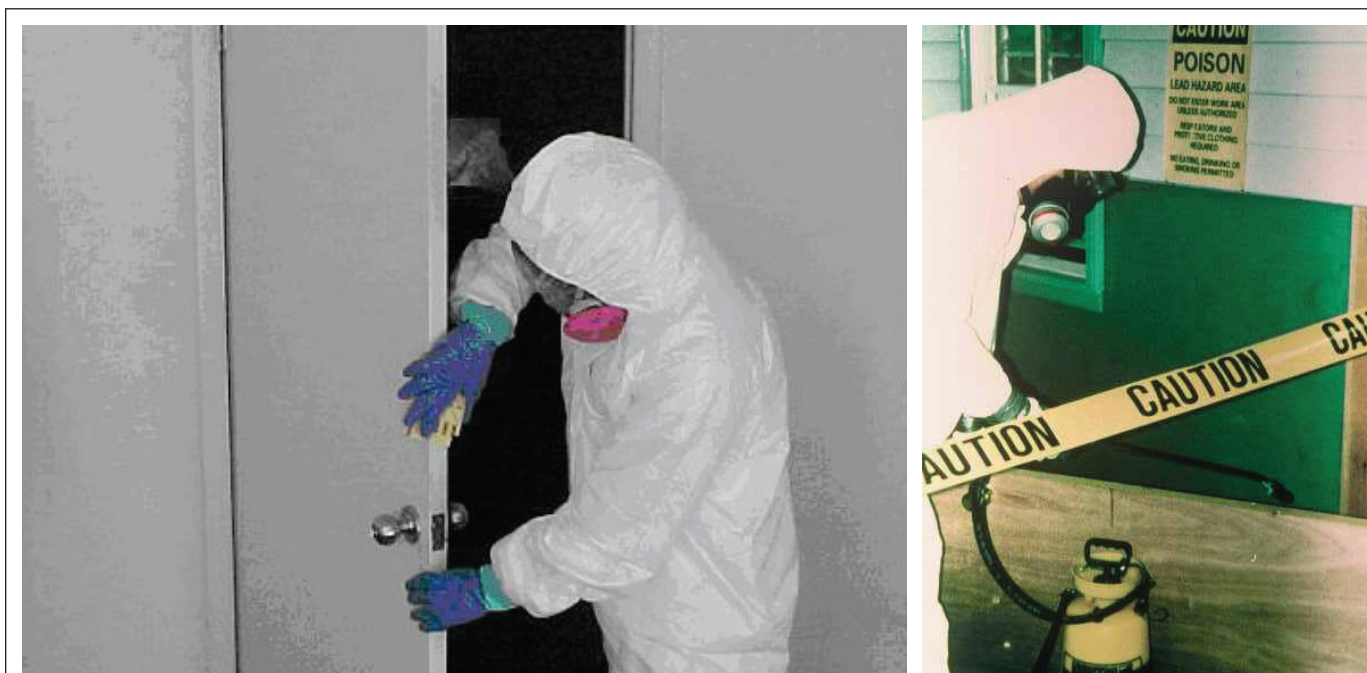
FIGURE 11.15 Stabilizing paint on doors: Wet planing (left) and wet sanding (right) deteriorated paint can create significant amounts of dust.
