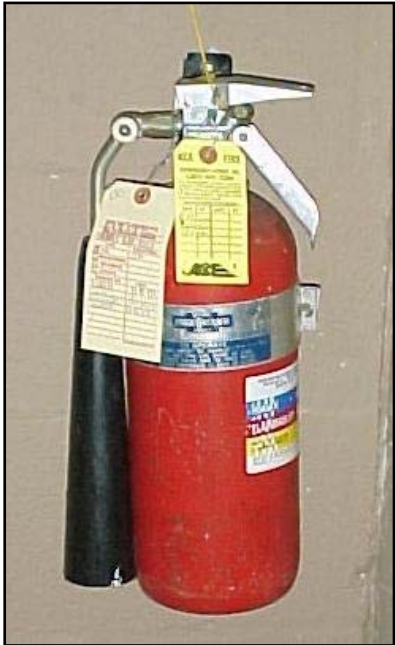
Figure 1: Carbon dioxide fire extinguisher
