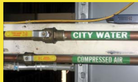
Hazardous energy sources
