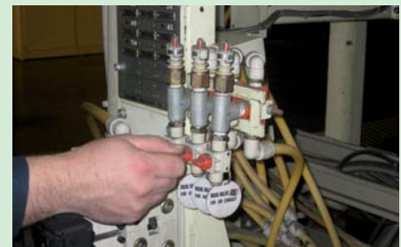
Bleeding air pressure by opening a valve
