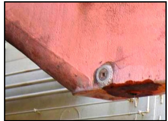
Figure 3. A vent plug indicating leaking product.
