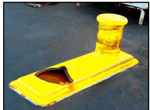
Figure 1. A hollow area under a mooring bitt.
