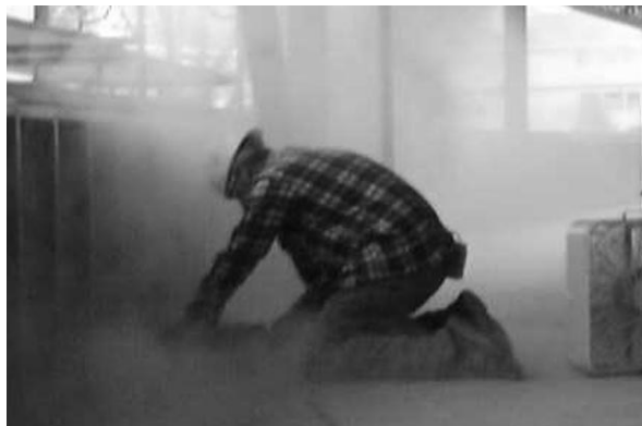
FIGURE 6. Surface Grinding: Rough walls, floors, and support columns were leveled using the flat surface of a 4.5 or 7 inch diameter surface grinder with an abrasive or diamond disk. At times this process takes an entire shift, while many times it was employed for only a small area or intermixed with patching.
