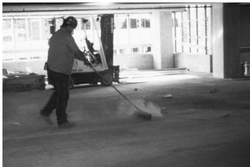
FIGURE 1. Cleanup: Cleanup involved the removal of construction debris, particularly settled dust, using brooms, shovels, and occasionally a backpack blower. There was often frequent interruption of the cleanup task to move obstructions out of the way.
