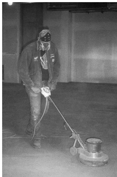
FIGURE 8. Floor Sanding: Floor sanding is a finishing process for smoothing cementitious floor underlayment products. The floor sander was a 16 inch diameter sandpaper disk and is operated from a standing position. This process was interrupted frequently to move obstructions out of the way.
