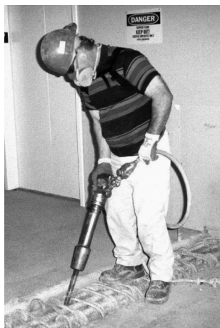
FIGURE 2. Hand Demolition: Handheld concrete demolition involved the use of a small jackhammer or reciprocating gun with interchangeable chipping or rivet busting head to remove excess concrete from overpours, splashovers or when concrete forms did not meet.
