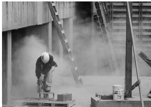
FIGURE 3. Concrete Cutting: Concrete block was cut using a handheld gasoline or a table-mounted masonry saw. The handheld saw was always used outside, and cutting was intermittent and always dry, whereas the table-mounted saw was used both inside and outside on scaffolding, usually cutting with at least some water spray to the blade and sometimes continuously for several hours.
