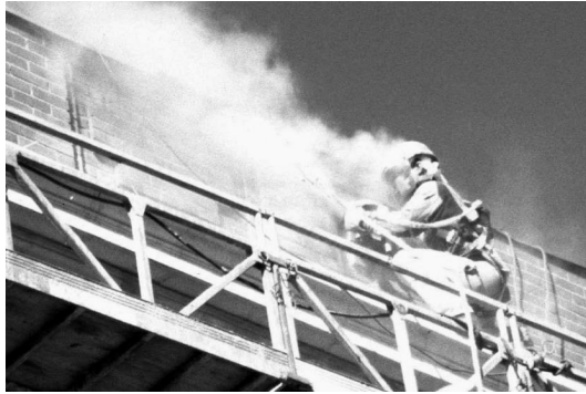
FIGURE 5. Tuck-Point Grinding: During masonry wall renovation, tuck-point grinding removes old mortar from between bricks, using a right-angle grinder. Usually, grinding occurs for half a shift and “tuck pointing” e.g. replacement of mortar, occurs for the remainder of the shift.
