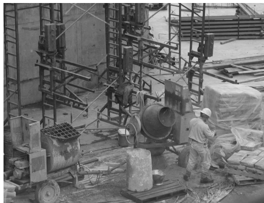
FIGURE 4. Concrete Mixing: Concrete, mortar, and grout are mixed, usually by the hod carrier on a brick mason crew. Typically mortar was mixed 3-4 times in a shift, with each session taking about 10 minutes. On two occasions, grout could not be delivered to the site and it was hand mixed, resulting in a fairly continuous period of mixing.
